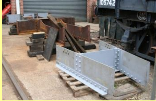
28/05/2011 - riveting completed in 'A' frame. In due course, the 'A' frame will be attached to the other end of the ladder frame (in the distance).and will have components such as the brake cylinder attached.
