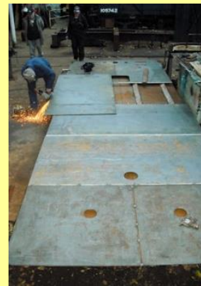
30/10/2010 - Substructure being prepared for welding. The image gives a clear idea of just how large the tender will be.
