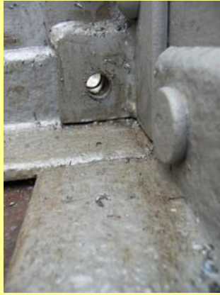
14/09/2011 - rivet holes in perfect alignment and ready for insertion of temporary bolts.
