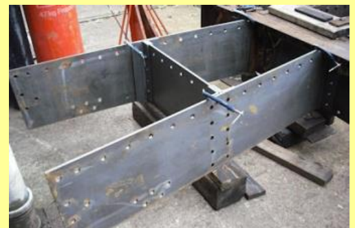
06/11/2010 - Lead stringers and spacer drilled and placed in position for riveting to the ladder frame
